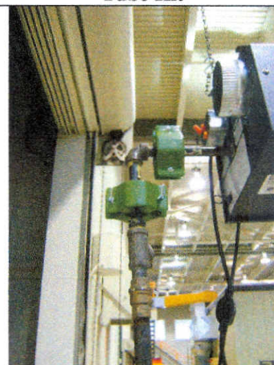
Get Green Device, installed
